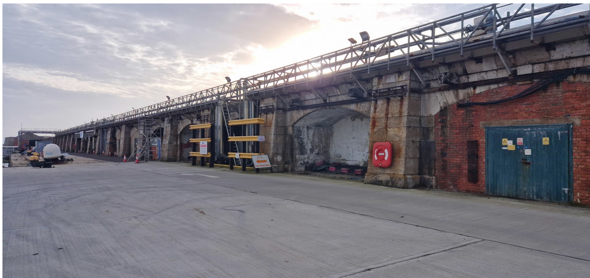
Figure 3 – PBUK fuel bunkering lines and hot oil lines along the jetty.
