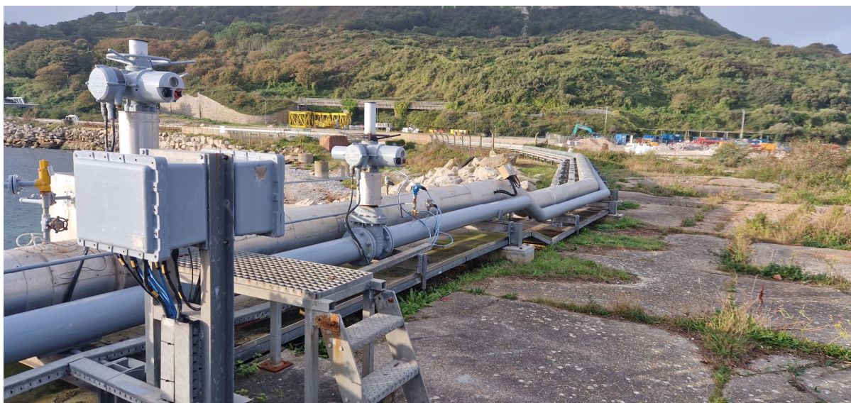
Figure 5 – PBUK fuel bunkering lines, hot oil lines and control next to Balaclava Bay.
