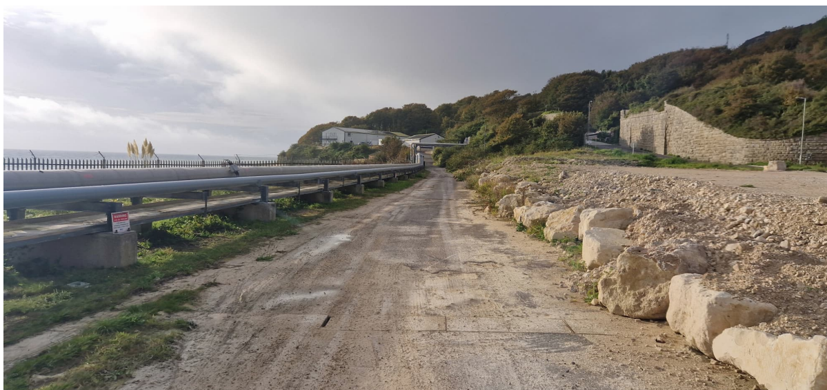
Figure 7 – PBUK fuel bunkering lines and hot oil lines next to Balaclava Road.
