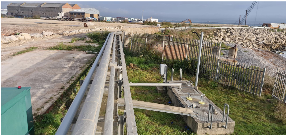
Figure 6 – PBUK fuel bunkering lines, hot oil lines, controls and sump next to Balaclava Road (PBUK control room, lube oil store and workshop in the background).
